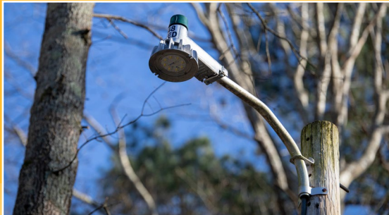
A102 | LED Security Light on Wood Pole
