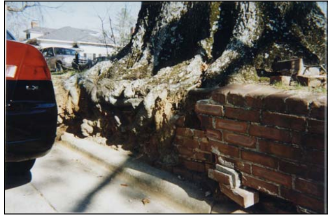
Photo 7. This willow oak (Quercus phellos) has damaged the a retaining wall and sidewalk as a result of its maturation. Large growth habit trees should be planted in sites with at least nine feet of grow space to prevent hardscape damage from occurring (W. North Ave.).
